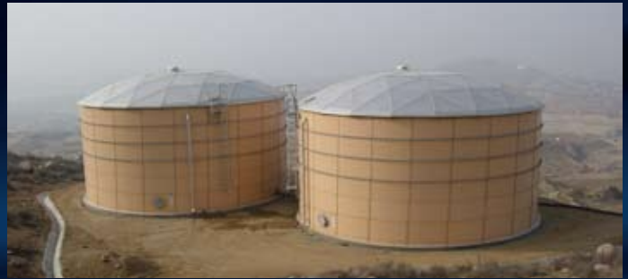
▲ Multiple potable ground storage tank facility.
