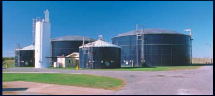
▲ Sludge stabilization and sludge storage facility.
